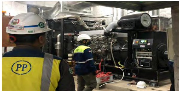
PT Pembangunan Perumahan - Dharmas Hospital Supply & Install (Genset, Fuel Tank 20.000 L) Austin Power System, Mitsubishi 1500 kVA x 2 Open
