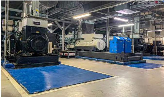
PT Dinamika Raya Prima - Data Center Supply, Install (Genset & Panel) Himoinsa, Mitsubishi 1250 kVA x 4 Open & Panel
