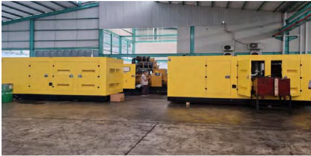
Hermina - Hermina Hospital Supply (Genset) Austin Power System, HD Hyundai 525 kVA x 10 Silent
