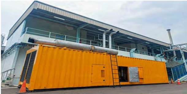
PT. Nippon Indosari Corpindo, TBK Rental Genset 1700 kVA & Load Bank 1400 kW
