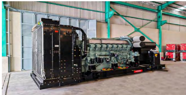
Inalum (Indonesia Aluminlum) - Inalum Factory Supply (Genset) Himoinsa, Mitsubishi 2250 kVA x 2 Open 3.3 KV
