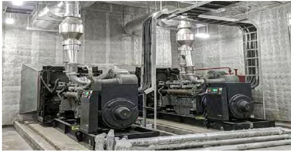
Anantara Uluwatu Ball Resort - Bali Supply, Install (Genset & Panel) Austin Power System, Perkins 800 kVA x 2 Unit
