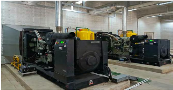
Wahana Dinamika Cakra - Data Centre Supply & Install (Genset, Fuel Tank) Austin Power System, Perkins 500 kVA x 2 Open
