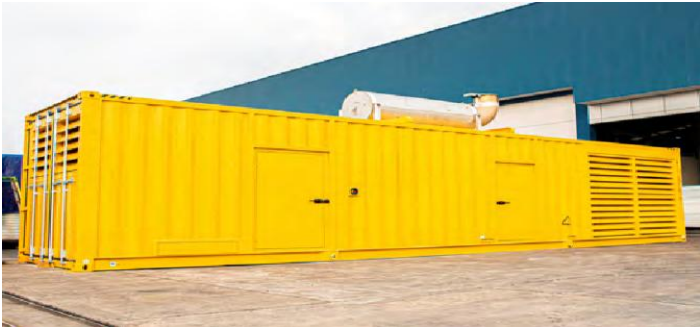
PT Hutama Karya - PLTU Suralaya Supply & Install (Genset) Austin Power System, MTU 3000 kVA Containerized
