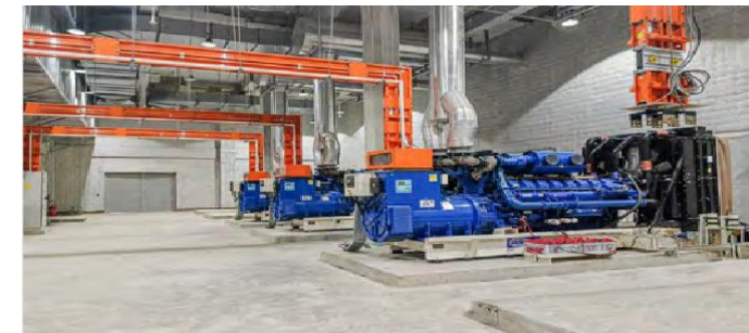
PT WIKA - Bandara Sultan Hasanuddin Makassar Supply, Install (Genset), Perkins 2000 kVA x 3 Open
