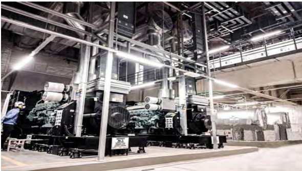
PT Kinden Indonesia - Mori Tower Supply (Genset & Fuel Tank 35.000 L) Himoinsa, Mitsubishi 2250 kVA x 4 Open
