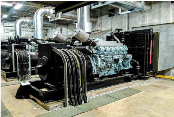
PT Indosat TBK - Data Center Supply, Install (Genset & Panel) Himoinsa, Mitsubishi 2250 kVA x 3 Open
