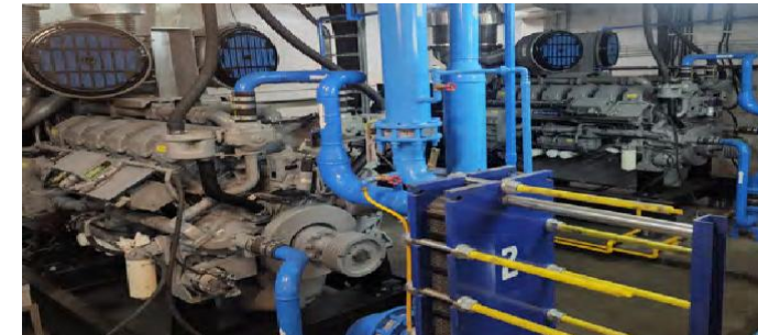
PT Bank Mandiri - Tunjungan Plaza Surabaya Supply, Install (Genset, Fuel Tank & Panel) Austin Power System, Perkins 1250 kVA x 2 Open
