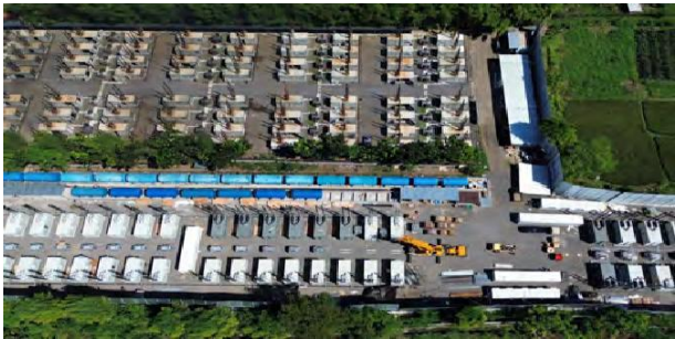
PT PLN - PLTD Supply, Install (Genset, Panel & Tank) Austin Power System, Cummins 1250 kVA x 148 Unit
