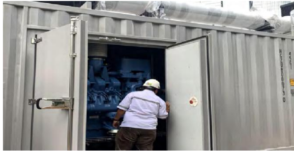
Summitmas - Summitmas Building 1 Supply (Genset) Himoinsa, MTU 2000 kVA Containerized
